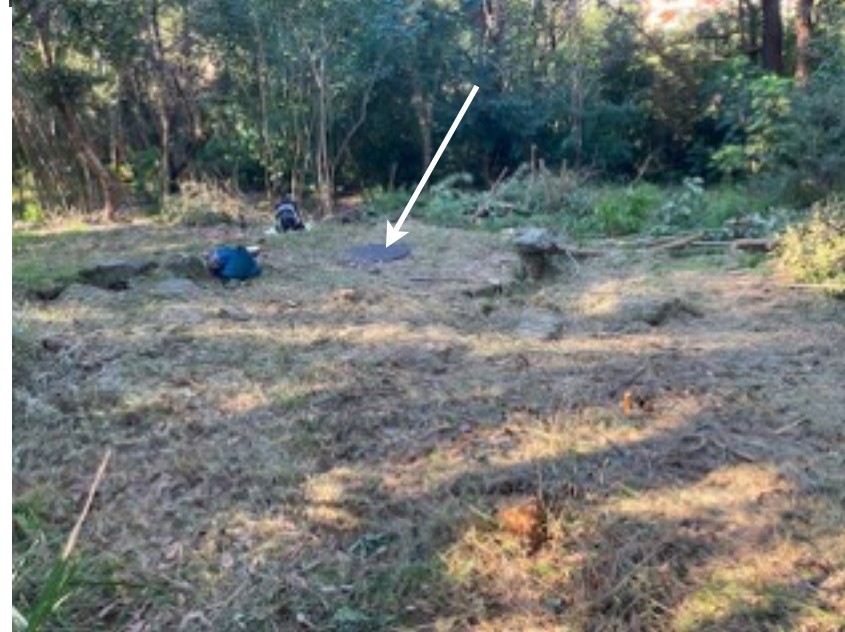
The area cleared around the access shaft (arrowed) - the REF claimed "no clearing or trimming of vegetation required." It has been stripped bare for about 10m x 8m.
